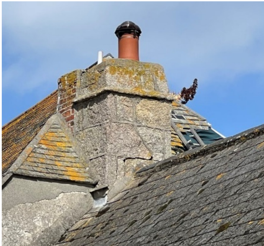
Fig 2: View of existing roof from Hugh Street, showing temporary weather protection.
