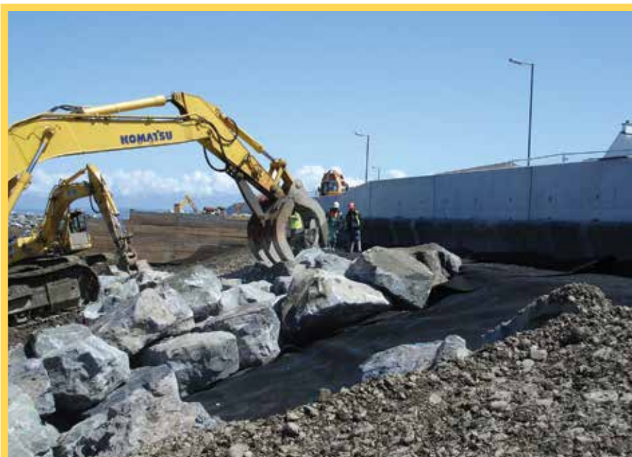
▲ Typical primary rock armour revetment installation directly on HPS geotextile. Location: Colwyn Bay.
