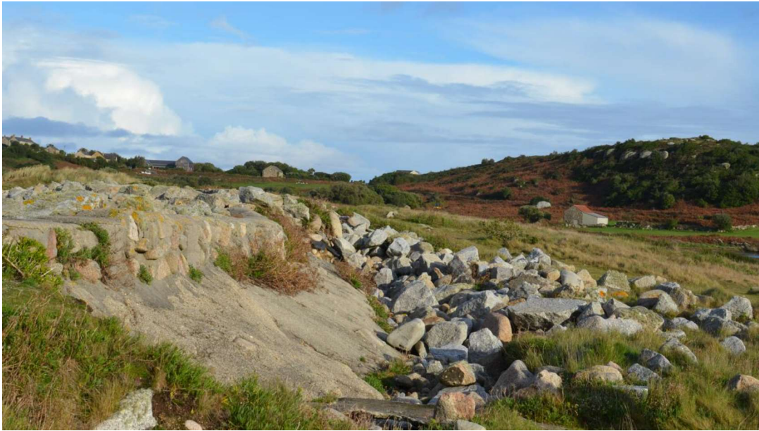
Figure 1-5: Dilapidated sea wall at Great Popplestone
