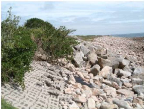
Figure 4-28: Damage to mattress and exposure of geomat (JLA 2014)
