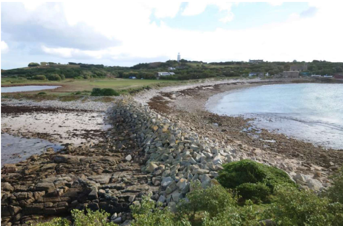
Figure 15: Former rail and boulder groyne from Ginamoney Carn to the point between Porth Coose and Periglis Beach.
