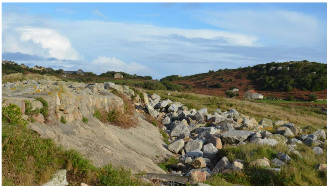
Figure 4: Run down sea wall at Great Popplestone.
