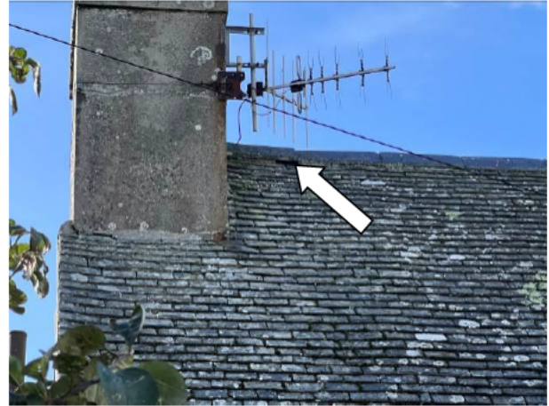
Photograph 2: Showing the roof structure – this is largely well-sealed with no gaps noted; however, occasional minor gaps are noted including the gap in the ridge highlighted.
