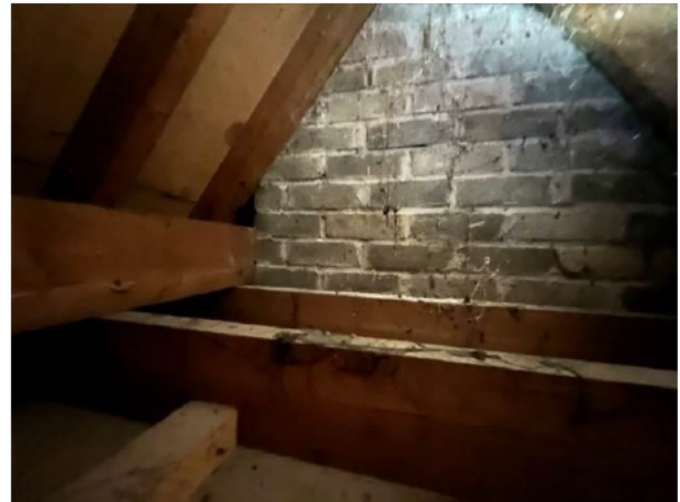
Photograph 4: Showing the loft space with boarding visible between the rafters.
