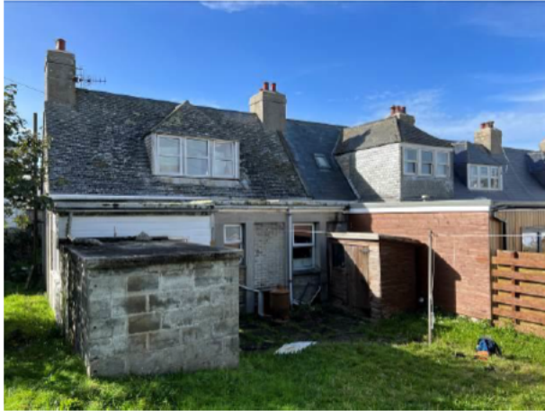
Photograph 1: Showing the property – the main property of 4 Porthcressa Terrace spans the length between the two chimneys on the left-hand side. The flat-roof extension can be seen in the foreground with the enclosed water-tank.
