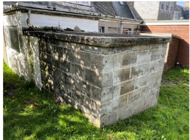
Photograph 6: Showing the enclosed water tank.
