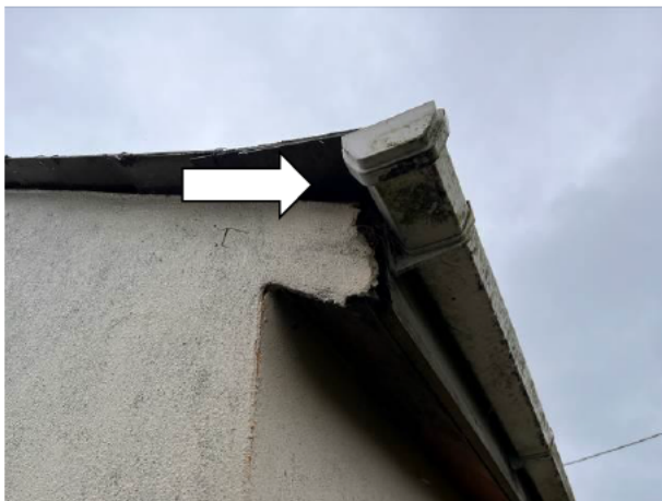
Photograph 5: Showing the minor cavity at the north-eastern corner of the building where a historic nest is present.
