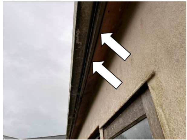
Photograph 4: Showing the soffits on the northern aspect – the minor gap between timbers is indicated.
