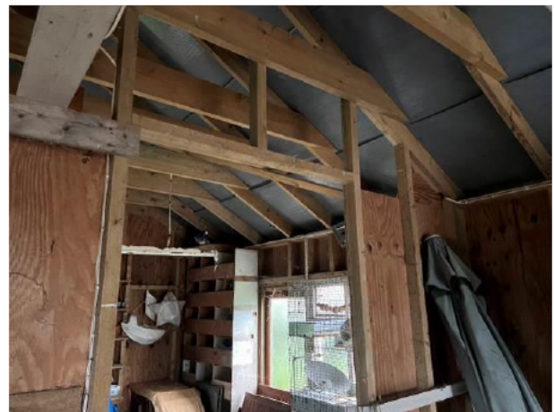
Photograph 6: Showing the interior of the property - the exposed studwork walls and well-sealed membrane above the rafters can be seen.
