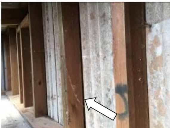
Photograph 5: Showing the internal wall timbers with corrugated sheets directly attached – minor gaps occur behind these.
