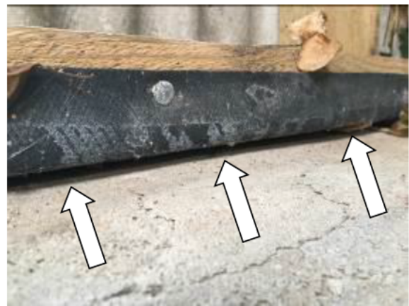
Photograph 4: Showing the minor gap occasionally present between the top of the wall and the timber wall plate.
