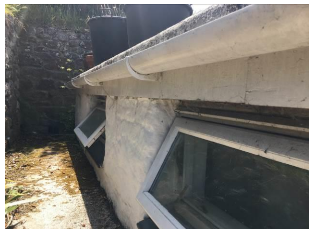
Photograph 6: Showing the fascia and guttering below the flat-roof section of the building (Section C) with well-fitted uPVC windows visible.
