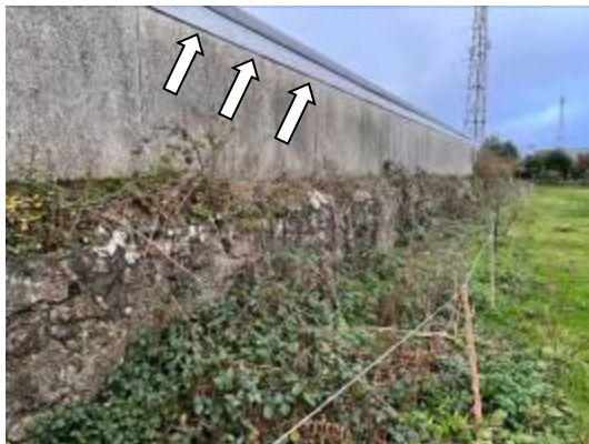
Photo 11 – Showing the garage immediately offsite adjacent to the stone wall on the western boundary. The gaps beneath the fascia are indicated.
