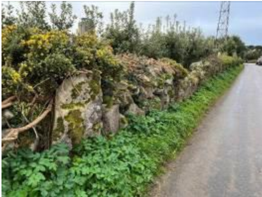
Photo 01 – Showing the northern stone boundary wall to the west of the site.
