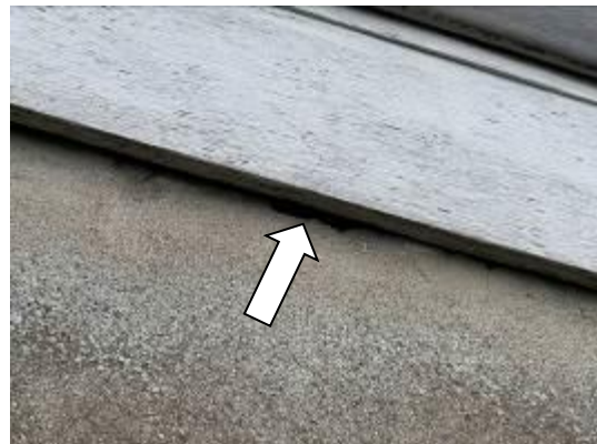
Photo 12 – Showing a closeup of the fascia board with a gap indicated.
