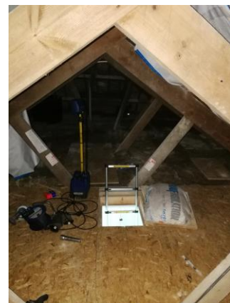
Photo 4. Showing roof void over main part of the house where works have been done
