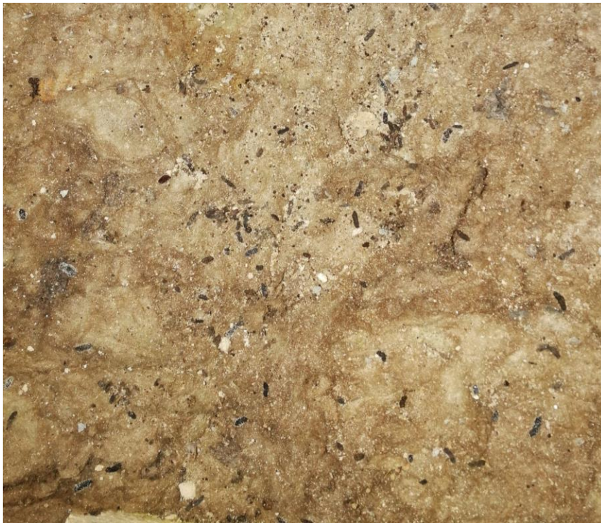
Photo 5. Showing a scattering of Common Pipistrelle droppings on the insulation
