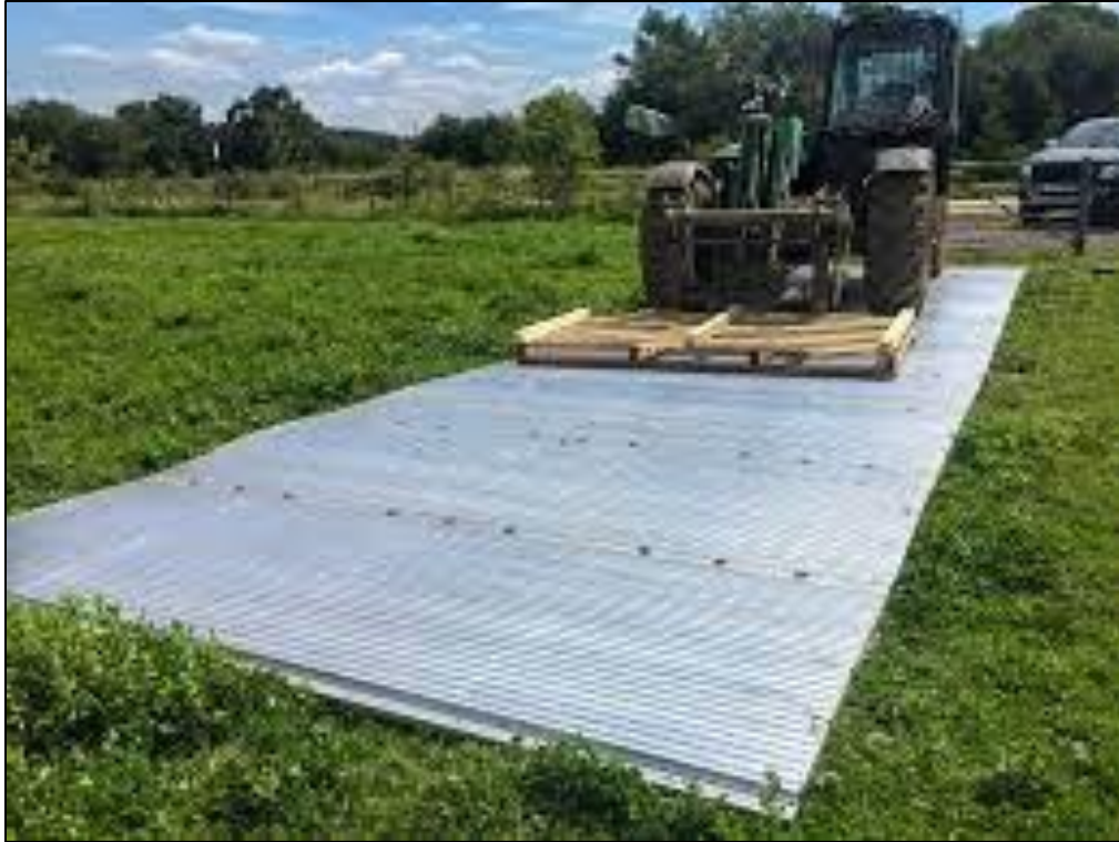
Figure 11 Example of the type of ground surface matting which will be used..
