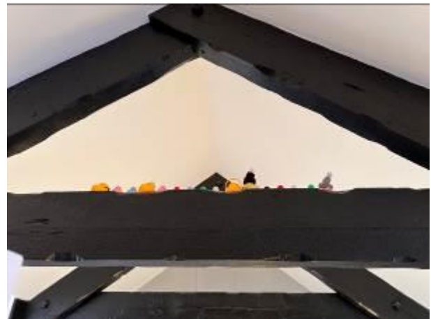
Photograph 4: Showing the top floor residential accommodation built into the apex of the roof throughout much of the span
