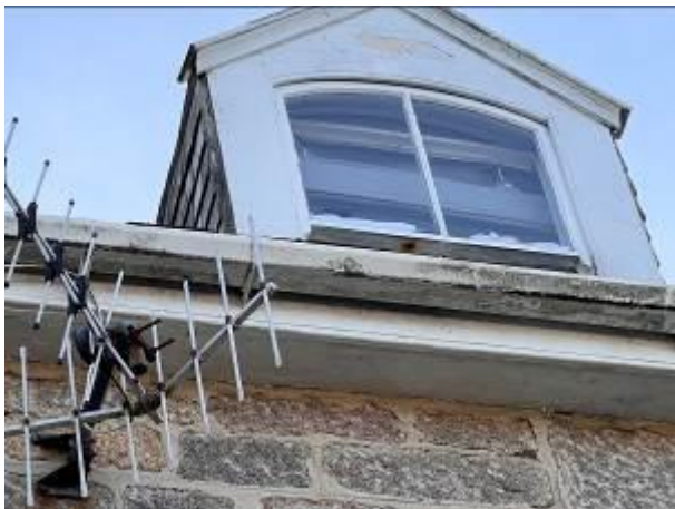
Photograph 3: Showing the well-sealed boxed soffit on the northern aspect with guttering attached
