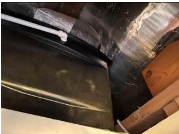
Photograph 5: Showing the water tank within the small loft void present in a portion of the roof. The insulation boards between the rafters can be seen.
