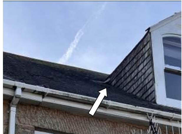
Photograph 2: Showing the minor lifted section of lead flashing around the junction between the dormer and the main roof
