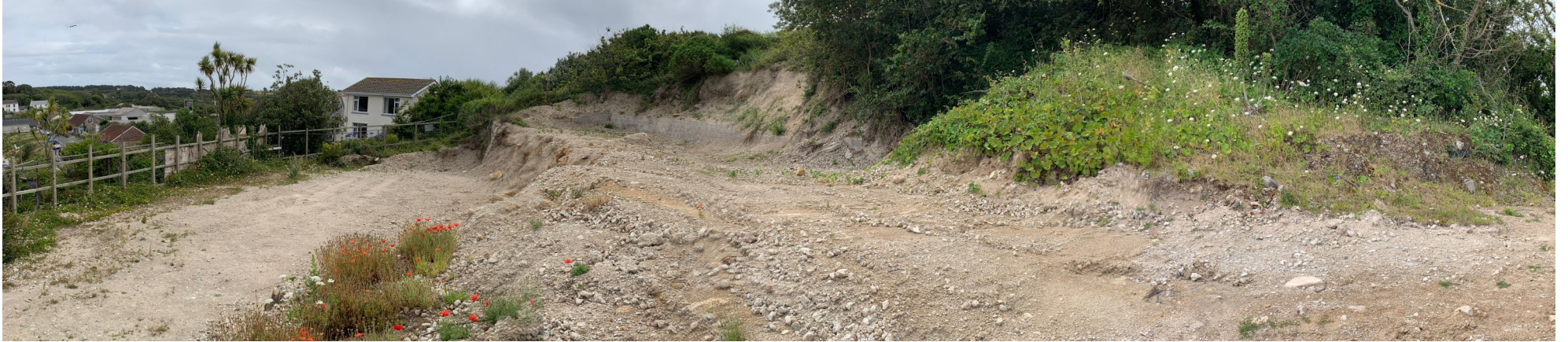
View C of the site looking East from the lower cleared plateau (post demolition).
