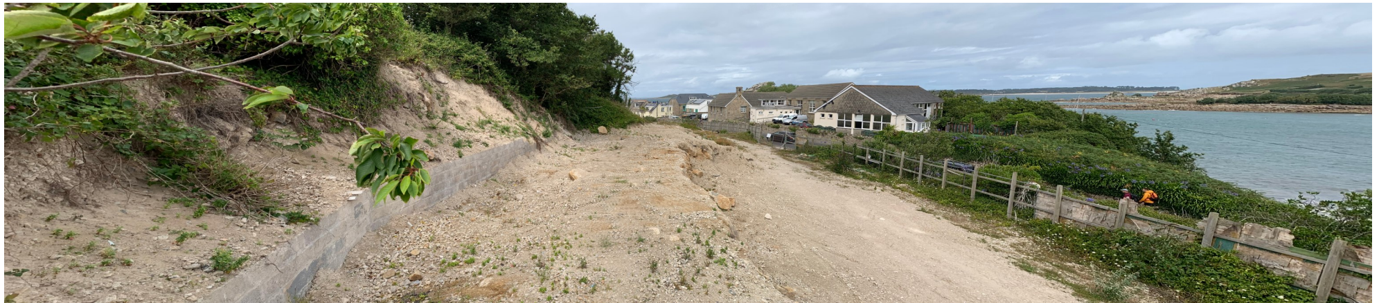
View D West facing view of the site from the lower cleared eastern half of the lower plateau (post demolition).
