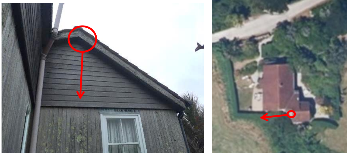
Figure 7: West elevation (left) and aerial view (right) of the south-east projection, showing emergence location of a single common pipistrelle bat on 25 th June 2020.
