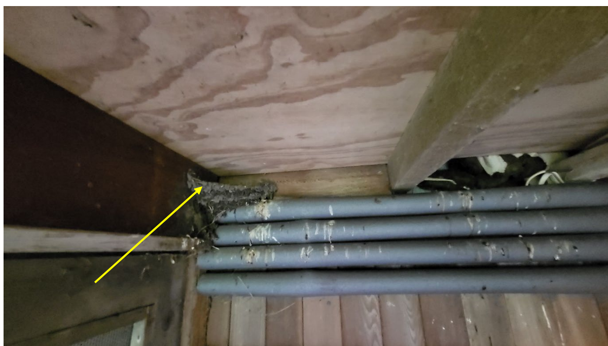
Figure 21: Swallow nest in the flat roofed boiler room on the north elevation
