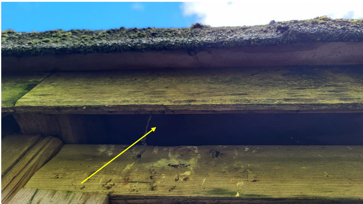
Figure 19: Gap between timbers allow access into the boiler room on the north elevation (yellow arrow)
