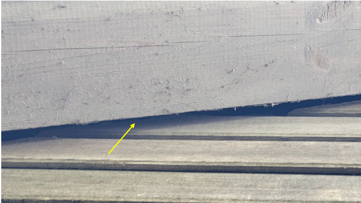
Figure 18: Gap behind soffit on the north elevation allowing potential access for bats (yellow arrow)
