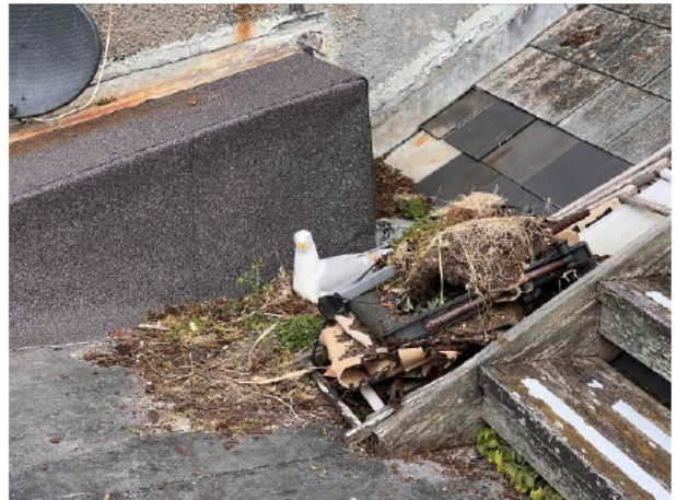
Photograph 4: Showing one of the herring gull nests on the flat roof of B&W B.
