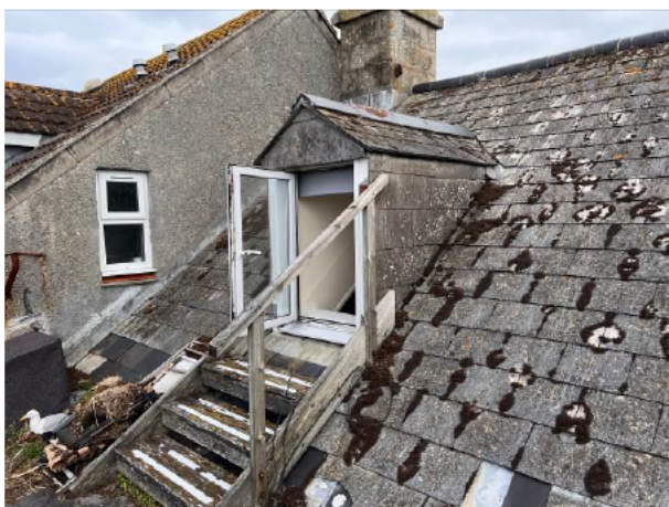
Photograph 5: Showing the access from the dormer of B&W A to the flat roof section B&W B. The synthetic tiles on the side of the dormers on this aspect are visible.
