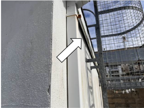
Photograph 13: Showing the gap behind the fascia on B&W B
