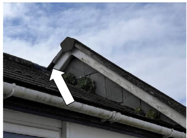
Photograph 12: Showing the gable of B&W D with missing pointing
