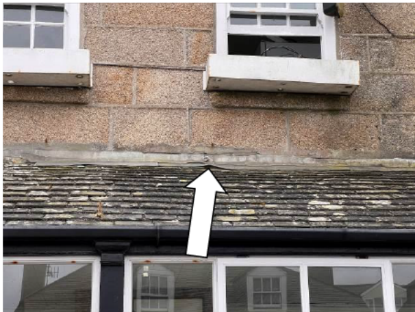
Photograph 17: Showing an example of lifted flashing where the roof of B&W F meets the main structure of B&W A
