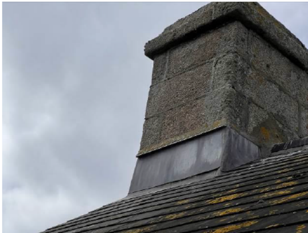
Photograph 3: Showing the lead flashing lining the junction between the chimney and the main roof of B&W A
