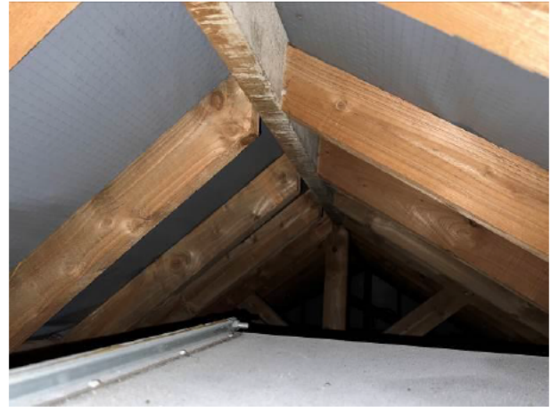
Photograph 8: Showing the interior of the loft space above B&W C with more modern felting.
