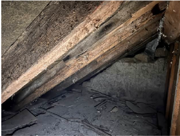
Photograph 1: Showing the interior of the roof void of B&W A at the eaves – the typical tar paper and poorly pointed gable can be seen
