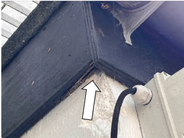
Photograph 15: Showing an example of a minor gap behind the fascia on B&W E
