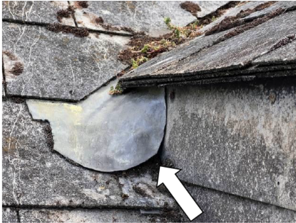
Photograph 7: Showing an example of the lifted flashing around the valley join between the dormer and the main roof on B&W A
