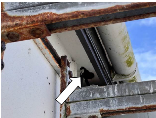
Photograph 11: Showing gaps in the soffit where services enter on B&W C
