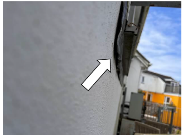
Photograph 10: Showing an example of lifted flashing beneath the window of B&W C
