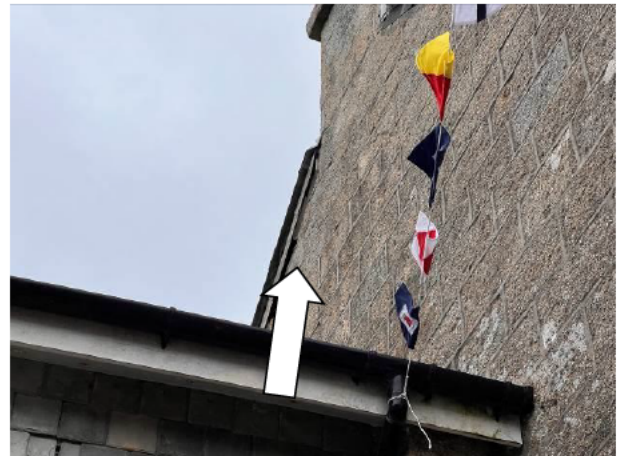
Photograph 18: Showing gaps in the gable verge of B&W A
