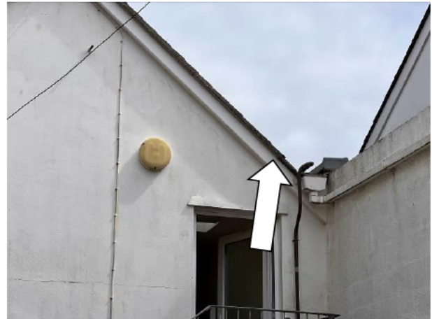
Photograph 16: Showing the gap in the verge pointing on B&W D
