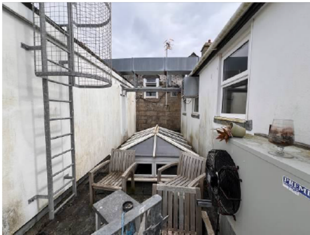
Photograph 9: Showing the 'courtyard' at first floor level created by the intersection of B&W A, B and C above B&W E.
