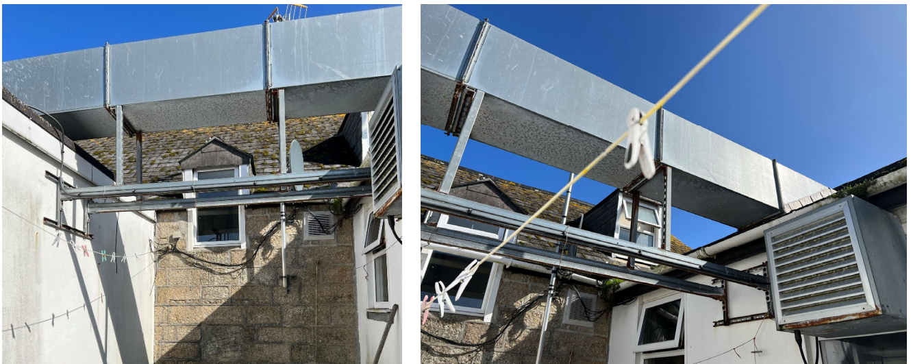
Figures 3-4: Existing extract ductwork
