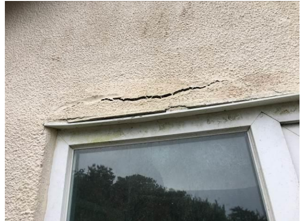
Photograph 2: Showing an example of the well-fitted window frames with no gaps or crevices. Cracks and damage in the render, as illustrated, are superficial and not suitable to support bats.
