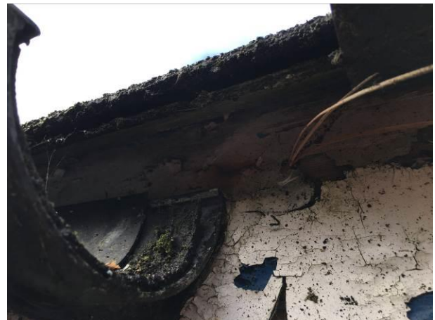
Photograph 4: Showing an example of the eaves where the guttering is displaced, demonstrating the lack of access for bats.
