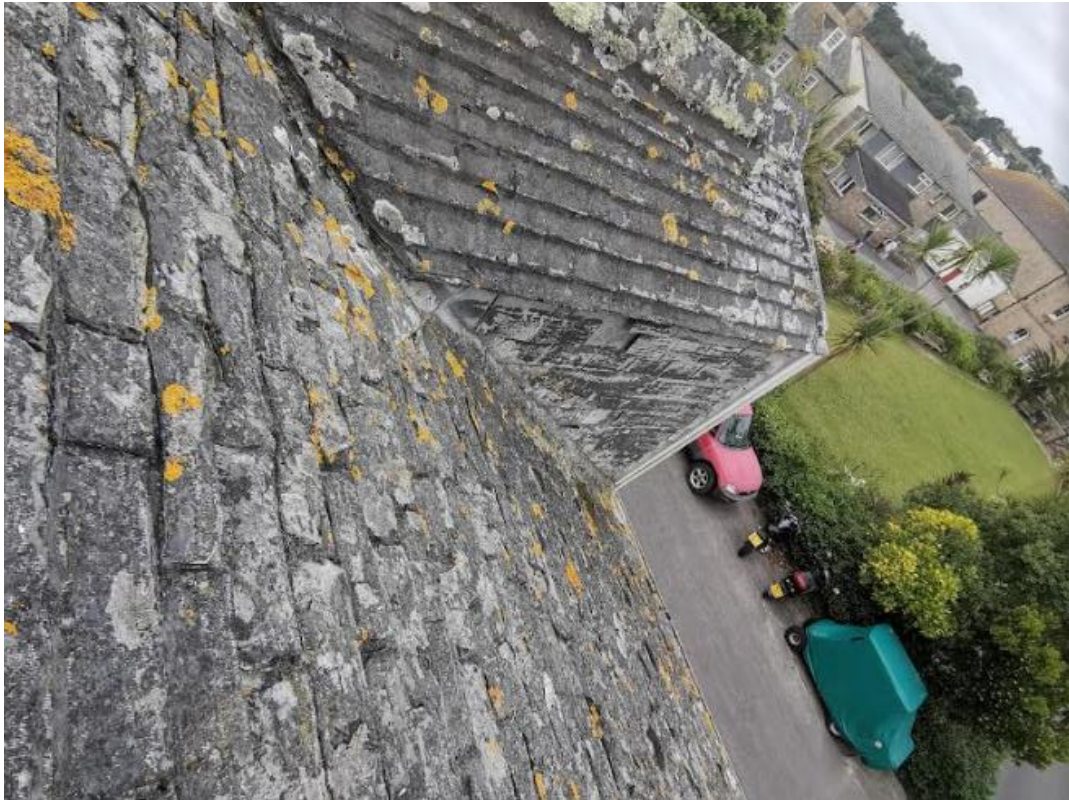
Pl.4: Detail of the front slope of the front range and the cheek and roof of a dormer.
