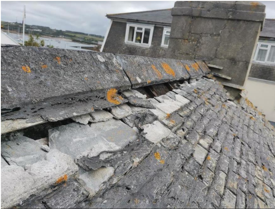
Pl.11: The roof of the rear range, showing obvious evidence of failure in the wet-laid scantle slate just below the ridge.
