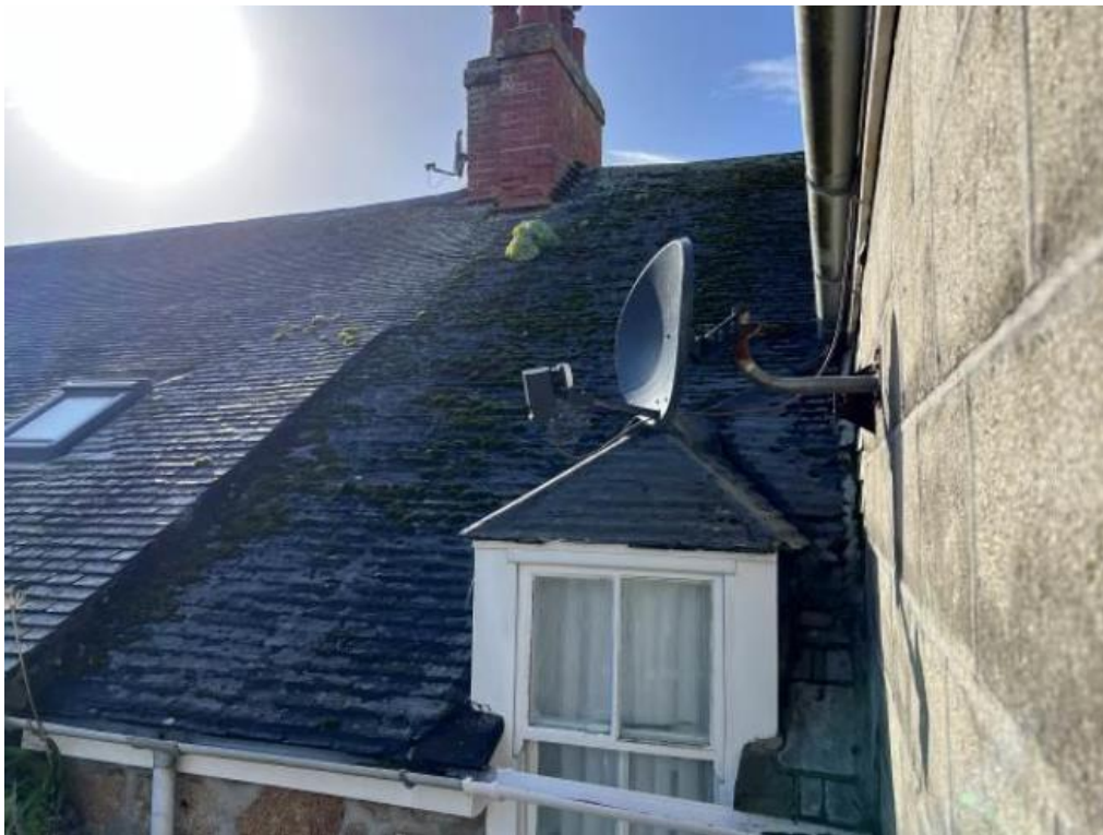
Pl.10: The southern end of the rear roof slope of the front range.
