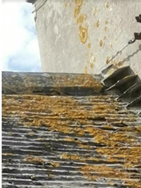
Pl.9: View of the northern end of the easter slope of the front range roof. Note slate slippage just below the ridge.
