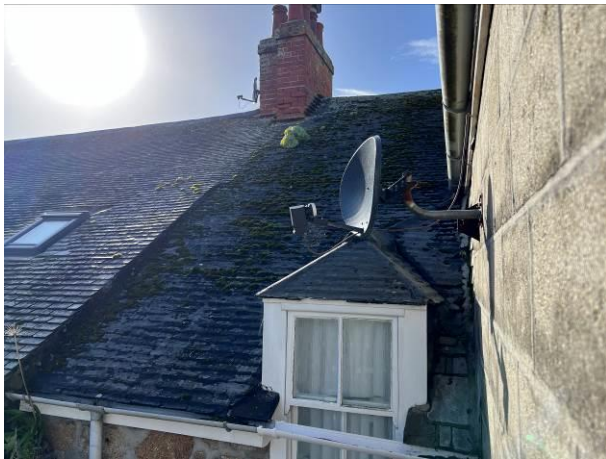
Photograph 3: Showing eastern pitch of the roof with the small dormer present. The surface covering above the scantle tiles can be seen.
