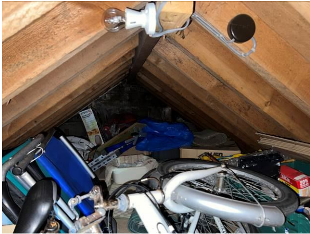
Photograph 1: Showing the loft space above the kitchen in the north/south aspect of the pitched roof.
