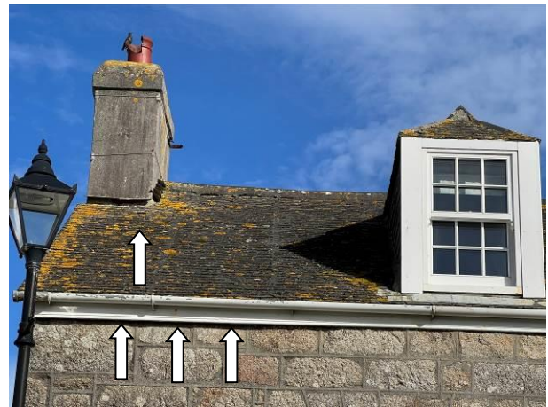
Photograph 4: Showing the western pitch of the roof – the gaps beneath the fascia are indicated along with an example of a gap beneath a tile below the chimney.
