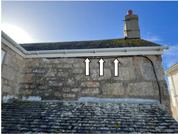
Photograph 7: Showing the single pitch #1 in the foreground with the gaps behind the fascia of the east-facing pitch indicated.
