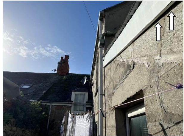
Photograph 8: Showing the gaps behind the fascia on single pitch #2.
