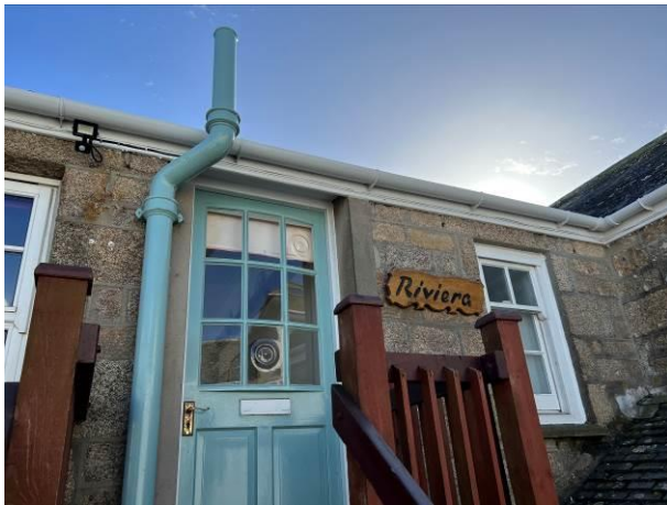
Photograph 9: Showing the entrance on the northern aspect – this is at the first-floor level. The fascias on this aspect are well-sealed.
