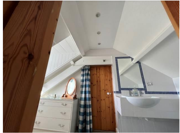
Photograph 2: Showing the rooms in the east/west pitched roof which are largely built into the rafters with the exception of minor sealed voids at the apex in one room.
