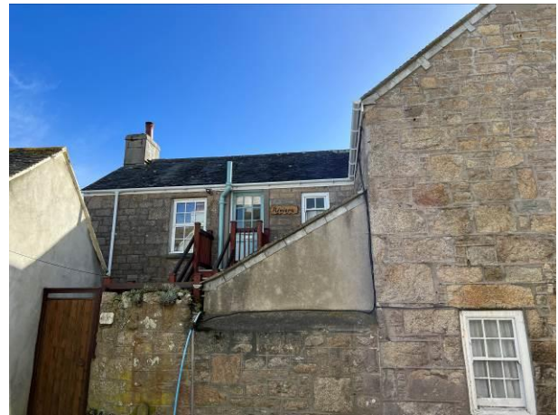
Photograph 10: Showing the northern gable of the pitched roof and the single pitch #1 in the foreground.
