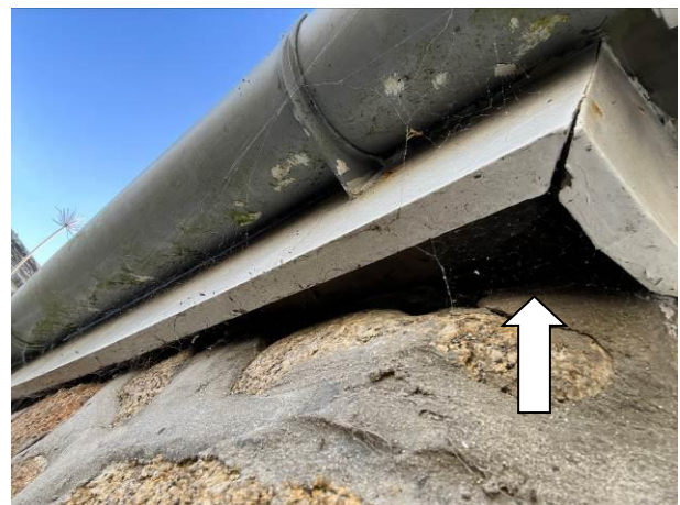
Photograph 6: Showing the gaps behind the fascia boards on the eastern pitch.
