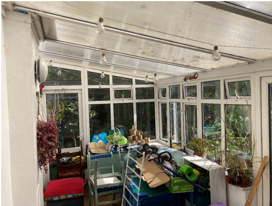
Photo 6. Interior of conservatory, SW elevation facing NE. Leaking water has caused blistering to paintwork and damage to oak flooring, while an electrical socket is no longer working and is isolated.
