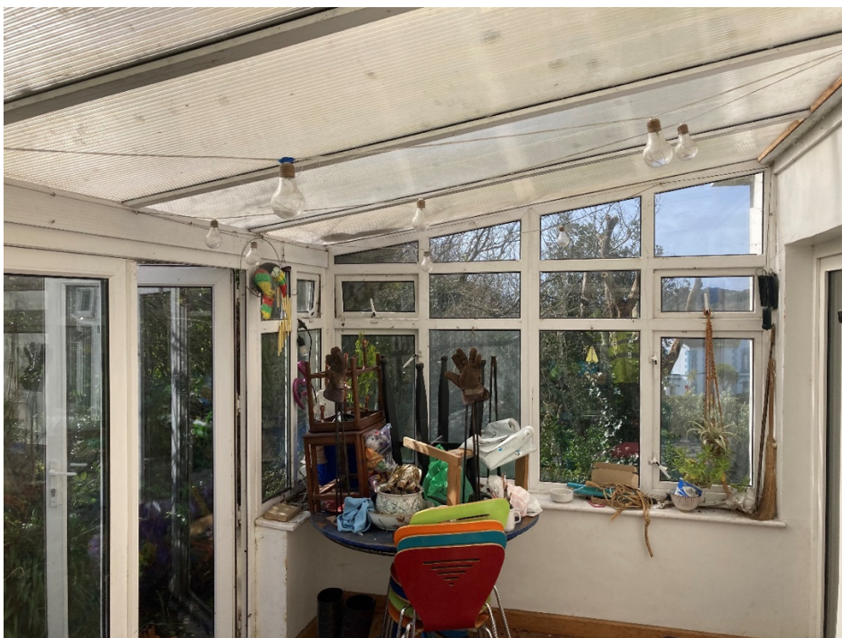
Photo 7. Interior of conservatory, NE elevation facing SW. Granite rocks holding roof down visible in lower left corner.
