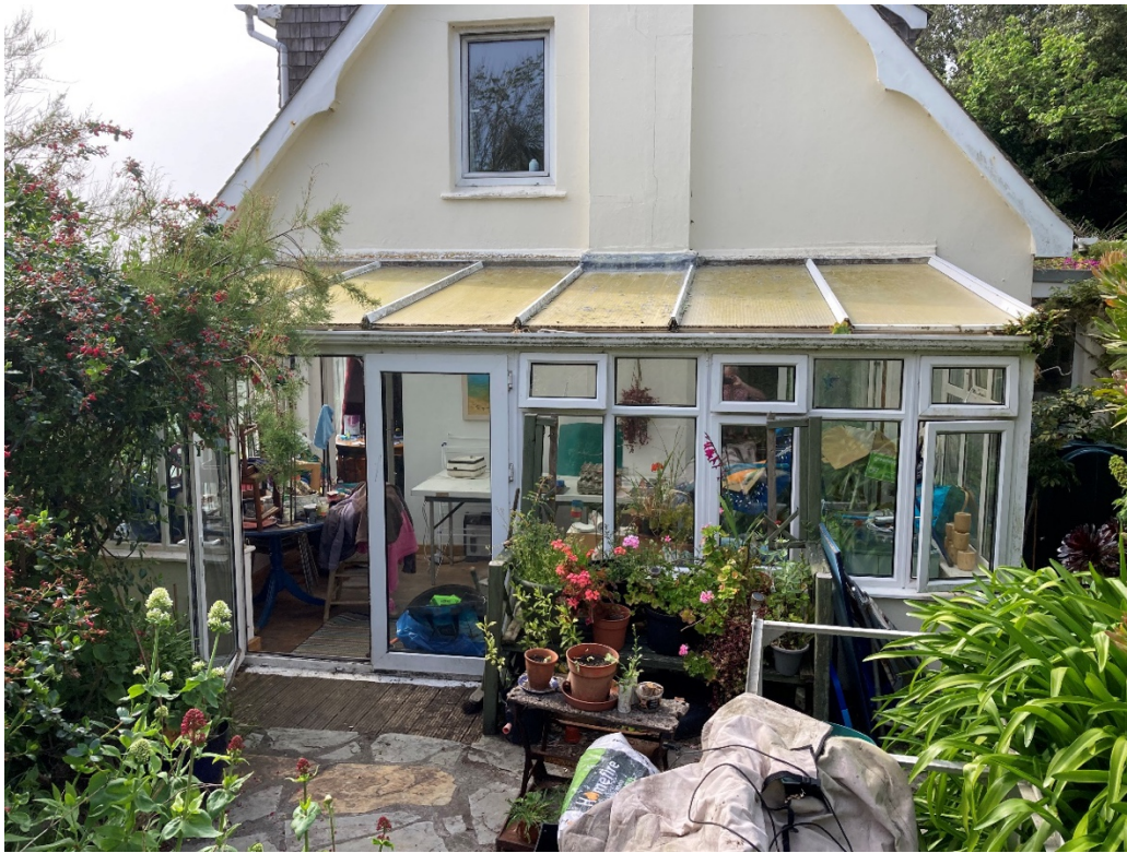
Photo 3. View of the conservatory from E elevation facing W. The conservatory roof is in very poor condition.
