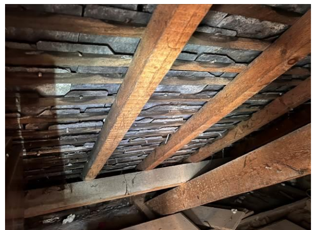
Photograph 6: Showing the interior of the unfinished portion of the eaves void – the wet-laid scantle tiles attached directly to battens are visible
