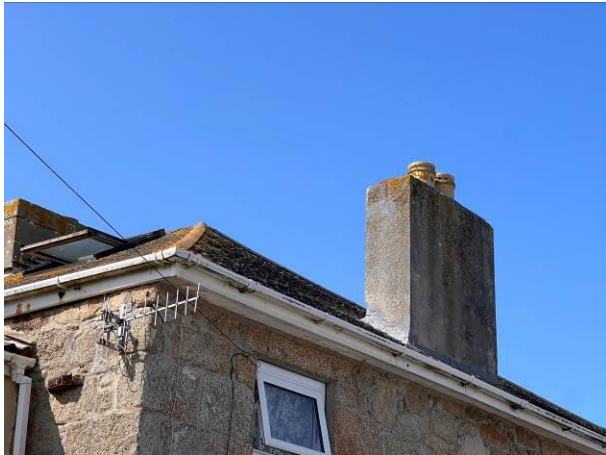
Photograph 1: Showing the northern aspect (with the chimney inset) – the tightly fitted boxed soffit is visible
