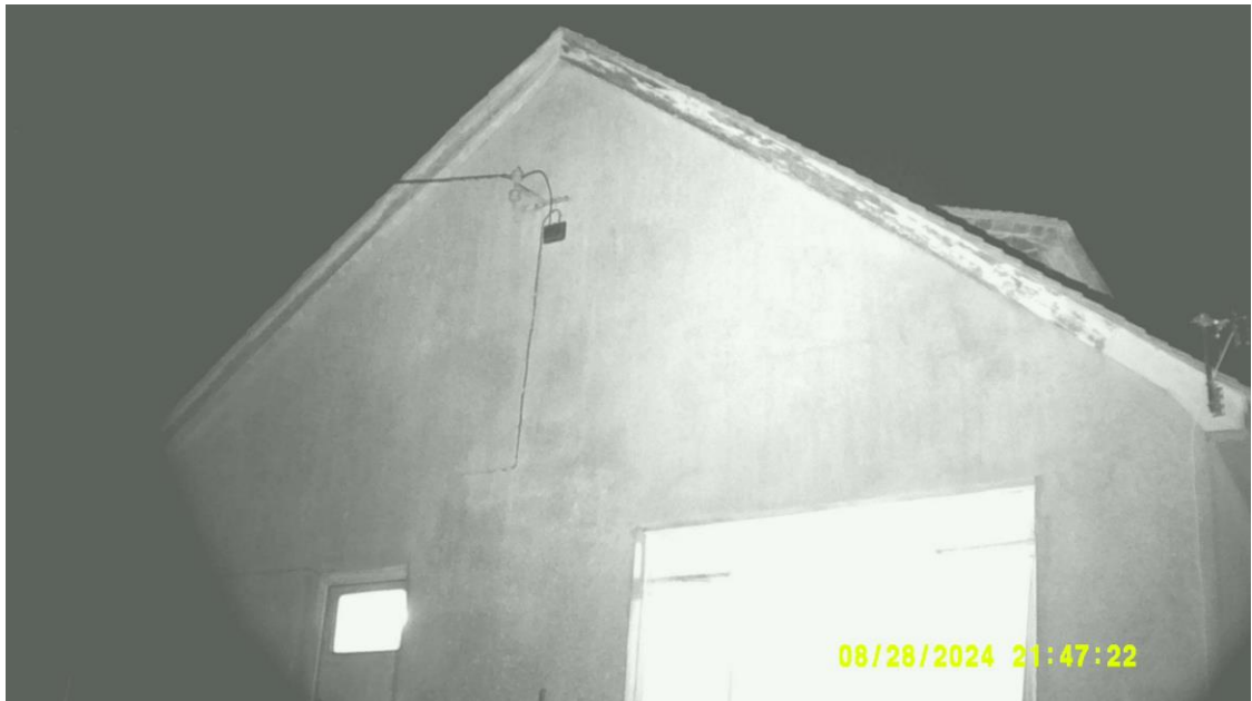
NVA1 – showing footage from the Nightfox Whisker at position S1. This is covering the south-eastern side of the building and includes all identified potential access features on this aspect.
