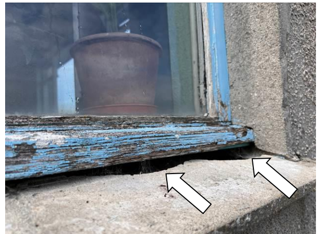
Photograph 4: Showing the potential access to the cavity wall below the window frame on the south-eastern corner of the property
