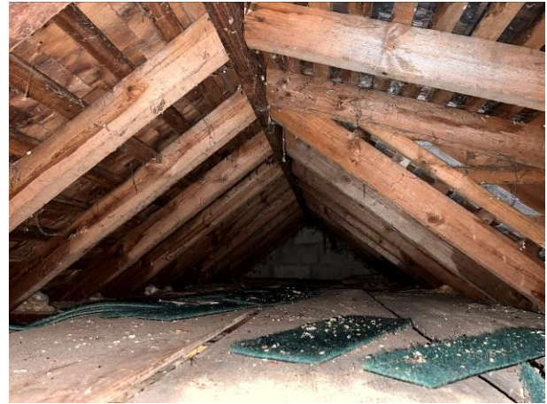
Photograph 8: Showing the apex void as viewed from the access hatch. The structural framework of the contiguous dormer void can be seen on the RHS of the image.
