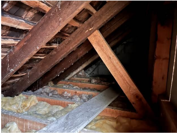
Photograph 7: Showing an example of the soffit voids within the property – the cedar shingles directly attached to the roof battens are visible
