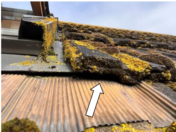
Photograph 3: Showing an example of the gap beneath a tile at the edge of the roof
