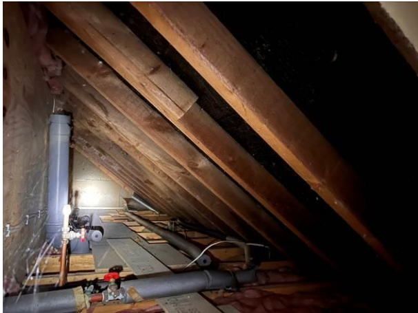
Photograph 1: Showing the internal boxed area at the eaves – this is an example of an un-finished void.
