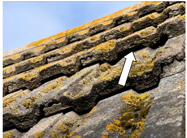
Photograph 4: Showing an example of the gaps at the intersections between tiles
