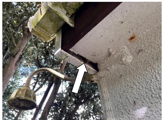
Photograph 6: Showing an example of a gap at the junction between the eaves soffit and the uPVC gable cladding.
