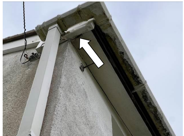
Photograph 10: Showing the gap in the soffit on the western gable with vegetation present indicating use as a nesting site.
