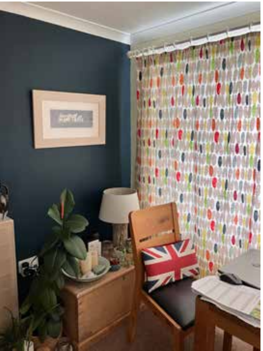
Existing area of wall in sitting room to be opened up through to kitchen
