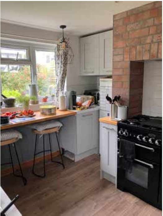
Existing kitchen window opening which will be removed to create walk through into new side extension. Wall cupboards to be removed and fridge relocated to create opening into sitting room
