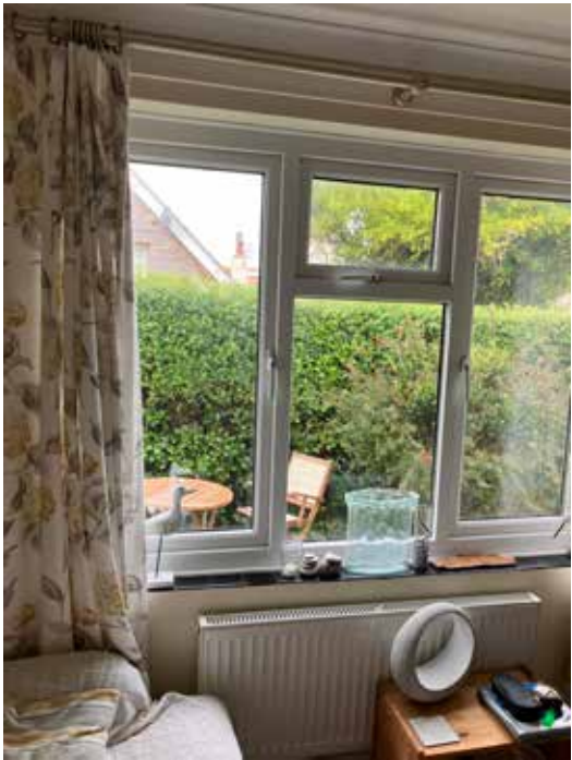
Existing front window to dining room which will be widened to walk through into the new extension
