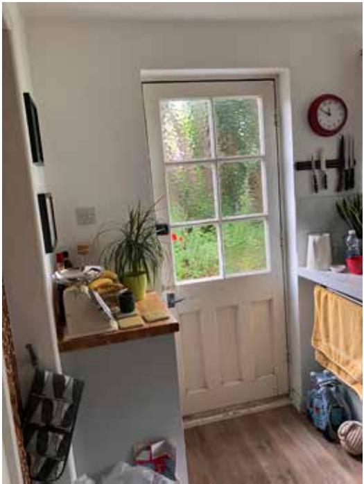
Existing kitchen door to be removed and turned into window with new worktop taken in front
