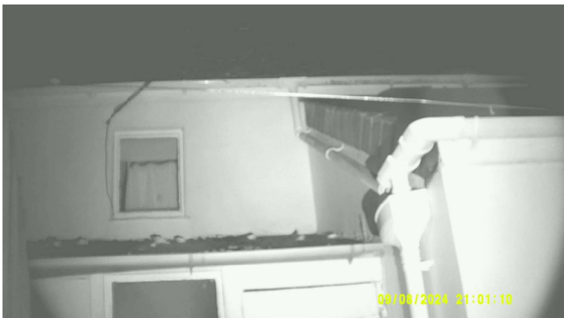
NVA2 – showing footage from the Nightfox Whisker on position S2. This is focussed on the fascias on the northern aspect of the property though the constraints of the site restricted comprehensive FOV in this location.
