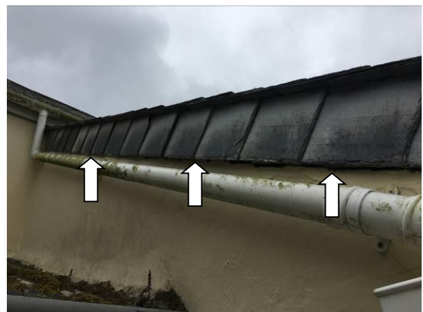
Photograph 6: Showing the drop-tiles on the gable of the Extension – gaps occur behind these tiles where indicated.
