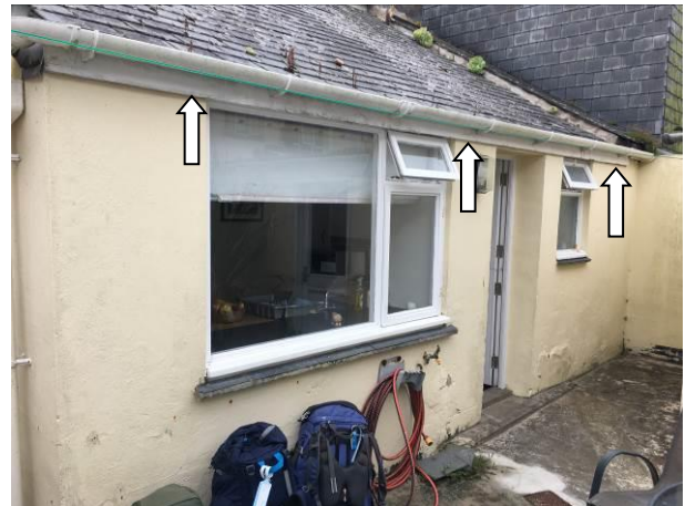
Photograph 4: Showing the front of the Extension – there are gaps behind the fascia boards on this aspect where indicated.
