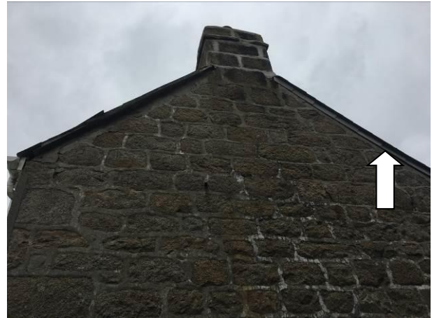
Photograph 2: Showing the gable end of the Cottage – there are minor gaps behind drop-tiles in places as indicated.
