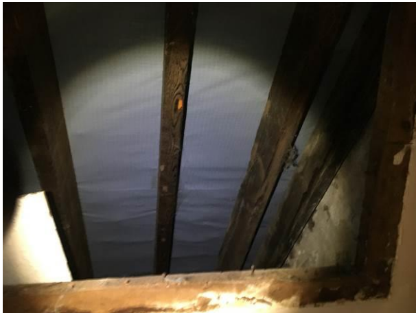
Photograph 9: Showing the roof structure within the minor loft space of the Extension.
