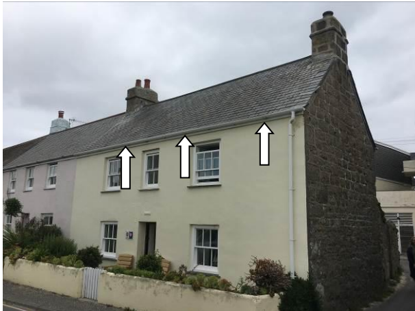
Photograph 1: Showing the front aspect of the Cottage facing Lower Strand. There are gaps under the fascia boards where indicated.
