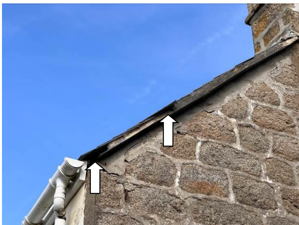
Photograph 11: Showing the slipped tile and missing verge pointing on the southern edge of the western gable.
