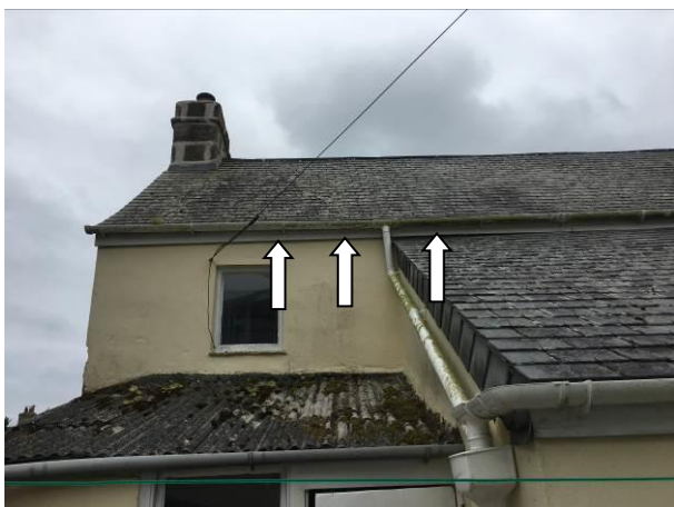
Photograph 5: Showing the rear aspect of the Cottage – the corrugated roof of the lean-to Utility can be seen at a lower height than the main Extension roof. There are gaps behind the fascias on the Cottage here as indicated.
