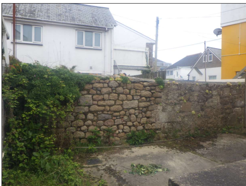
Plate 3: Two phases of stone wall bounding the existing pumping station site, view to southeast
