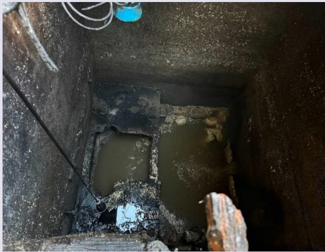
Wet well chamber
