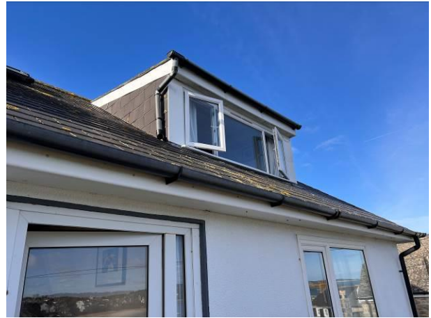
Photograph 2: Showing the front aspect of the property with one of the dormers present in the northern pitch visible
