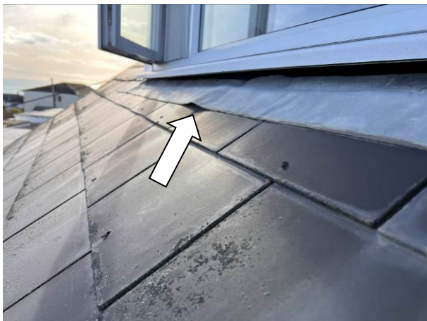
Photograph 5: Showing an example of the minor lifted flashing where the existing dormer meets the roof
