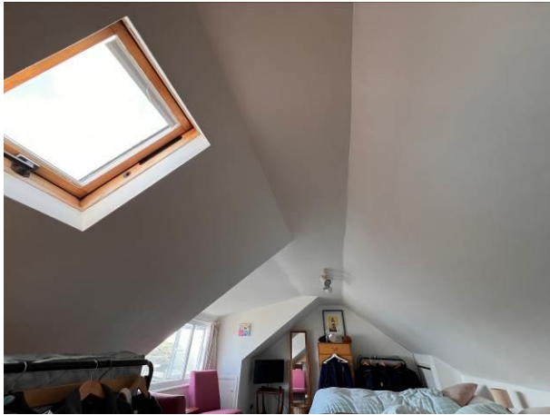
Photograph 7: Showing the interior of the loft conversion – the sealed apex void is visible
