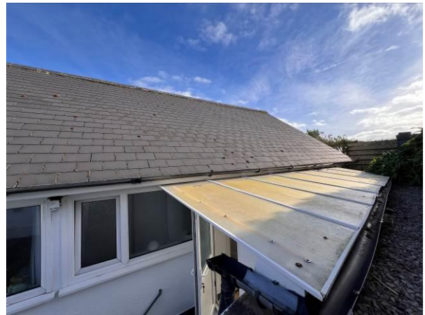
Photograph 4: Showing the rear southern pitch of the roof with the lean-to structure visible
