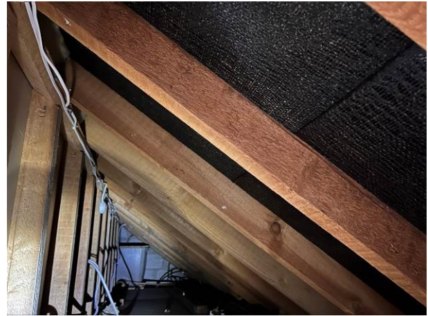
Photograph 8: Showing an example of the eaves storage with well-fitted roofing felt visible above the timber trusses
