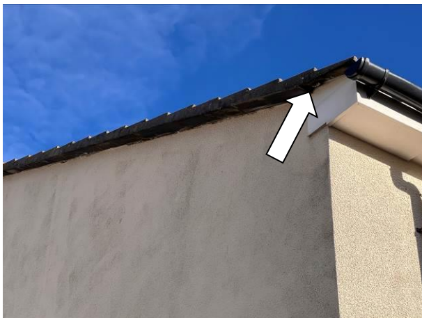
Photograph 5: Showing the location of the missing pointing on roof verge of the western gable
