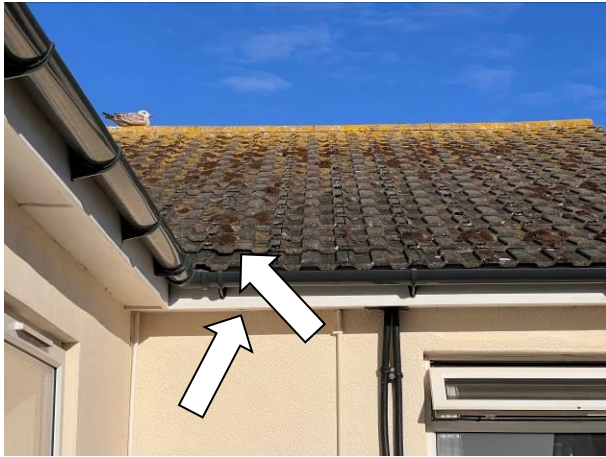
Photograph 7: Showing the southern aspect of the property – an example of lifted tiles is indicated by the upper arrow - whilst the lower arrow identifies the pipe hole in the soffit on this aspect.
