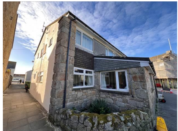
Photograph 4: Showing the eastern gable of the property with the mono-pitch roof structure visible on the northern frontage.
