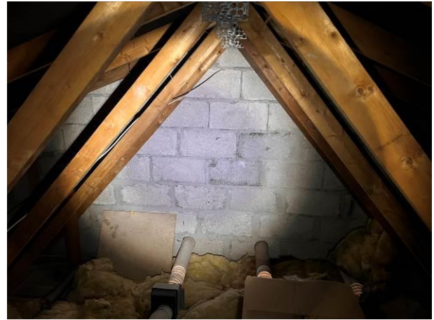
Photograph 8: Showing the interior of the loft space – the breeze block gable wall can be seen with the timber truss framework in the foreground.
